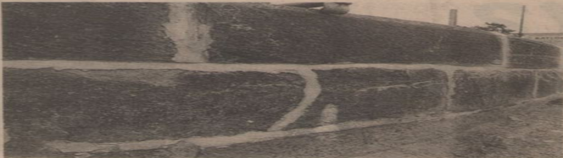
The cracked stone joined with a curve of cement on Hampsthwaite's river bridge. (R1067/20A)
