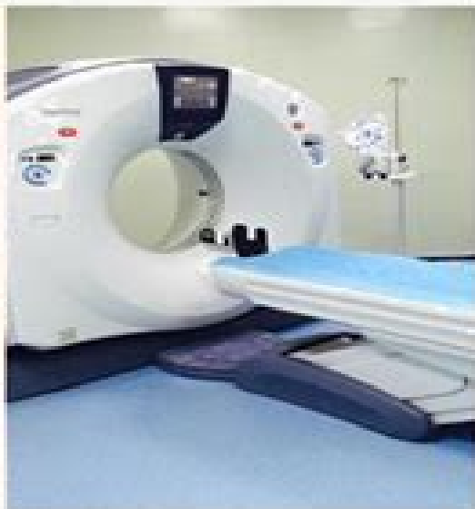
Hospital CT Room
