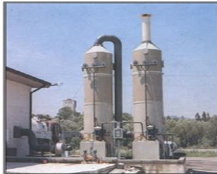
DOUBLE STAGE DEODORIZATION SYSTEM
