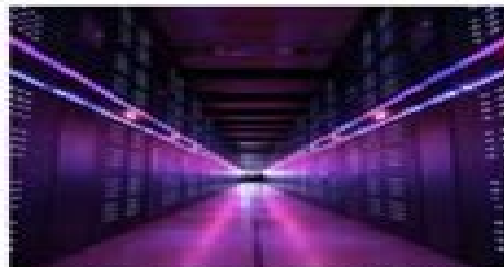
Tianhe computing platform
